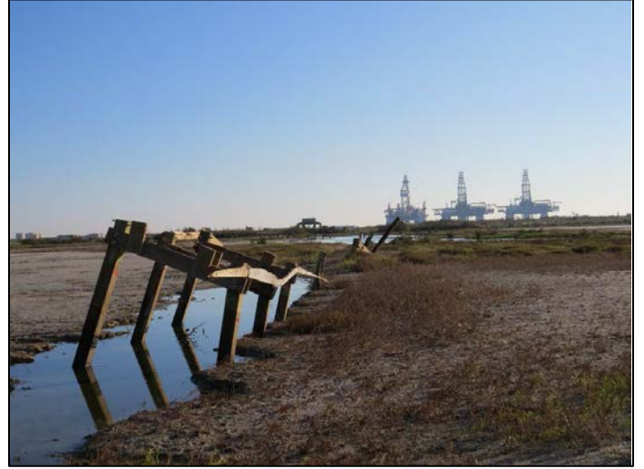
Remains of boardwalk, which was almost completely destroyed.
