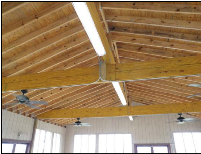
Above: Lights and Fans in Classroom
