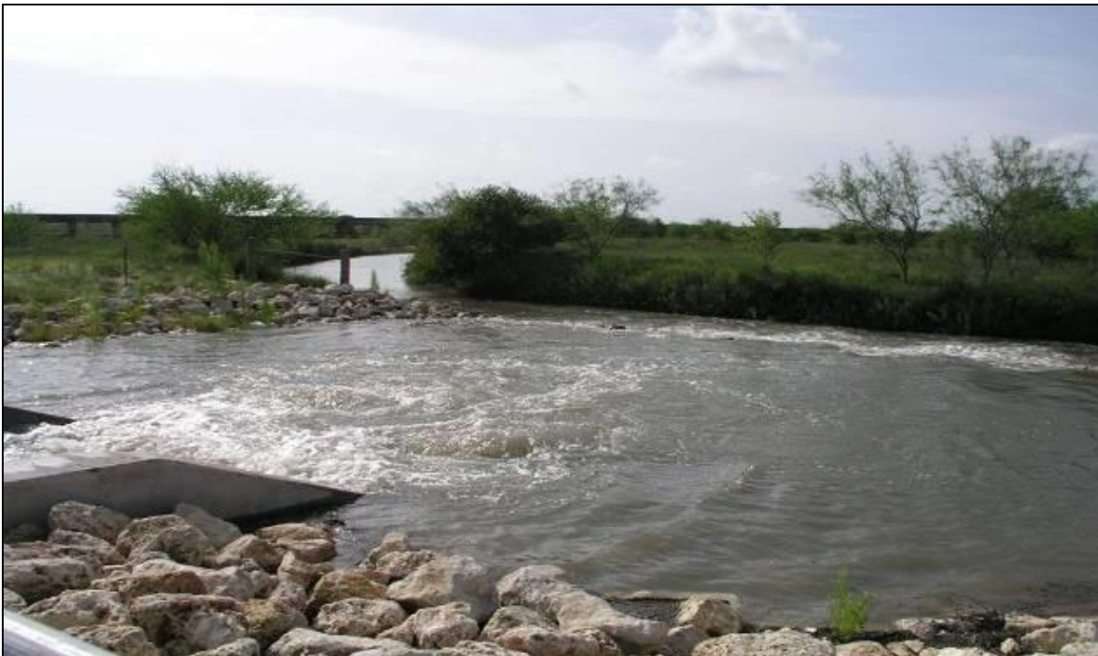
Figure 2. Rincon Bayou Pumping facilities A) the intake pumps located on the Nueces River above the Calallen Dam and B) the pipeline outfall in the Rincon Bayou. Photos taken by Jace Tunnell.
