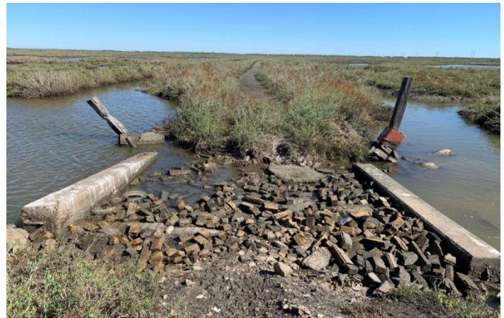
One of three culverts destroyed by Hurricane Harvey.
