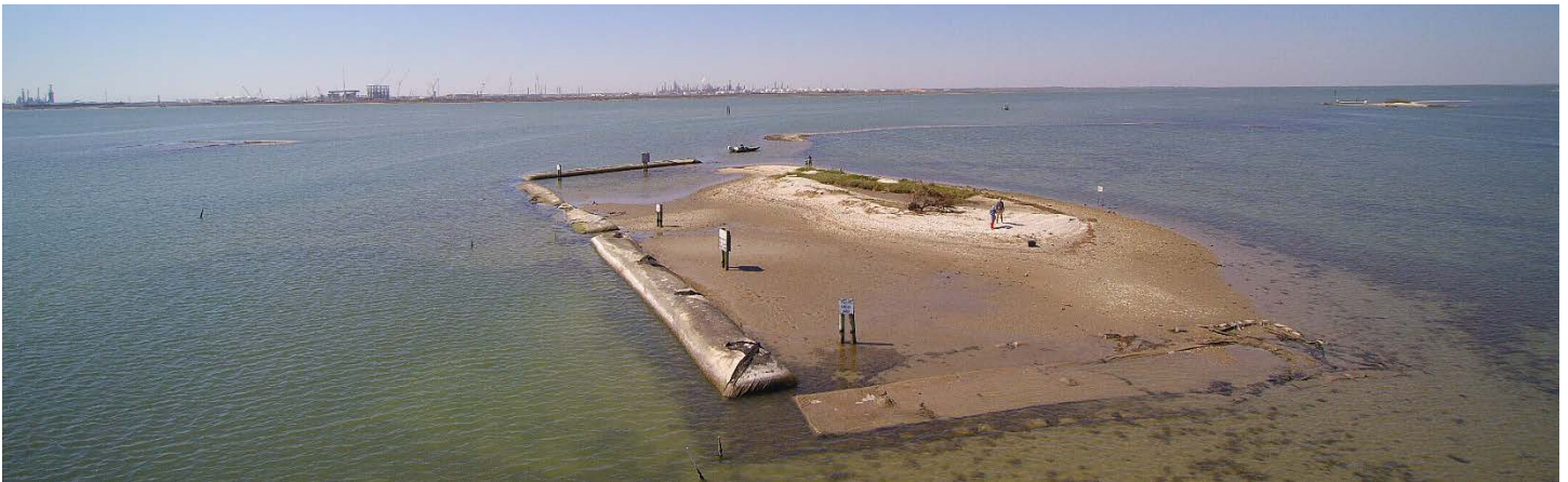
Birds eye view of one of the islands to be restored showing failed geotubes and eroded shoreline.
