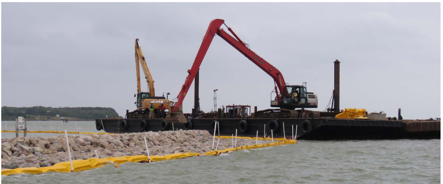
Construction begins with placement of the rock breakwater around one of the islands.
