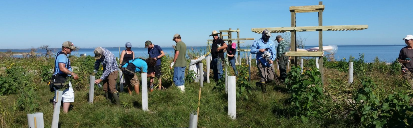
Workday on Second Chain in Aransas Bay, installing nesting platforms and signage, and planting native vegetation.
